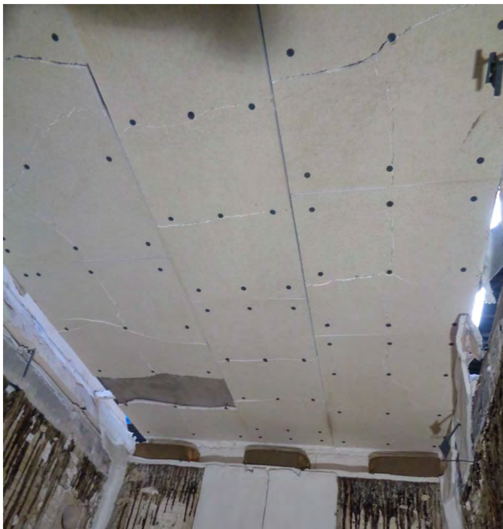
Photo L Exposed side after the test and cooling down.
