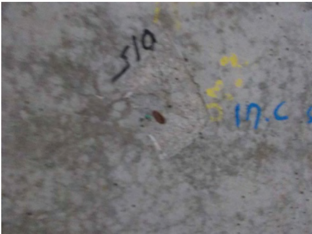
Photo I (up) Photo of the thermocouple on the exposed side of the slab - Section S9. Photo J (down) Photo of the thermocouple on the exposed side of the slab - Section S10.
